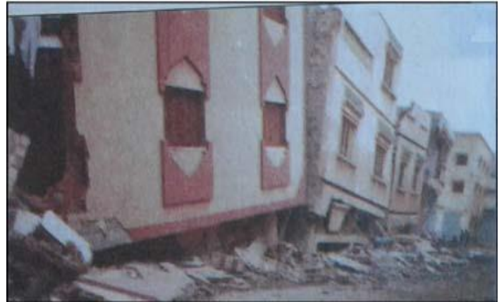
Picture 4a. Earthquake Damage in Al Hoceima, Imzouren (24 February 2004) Morocco (p 21).
