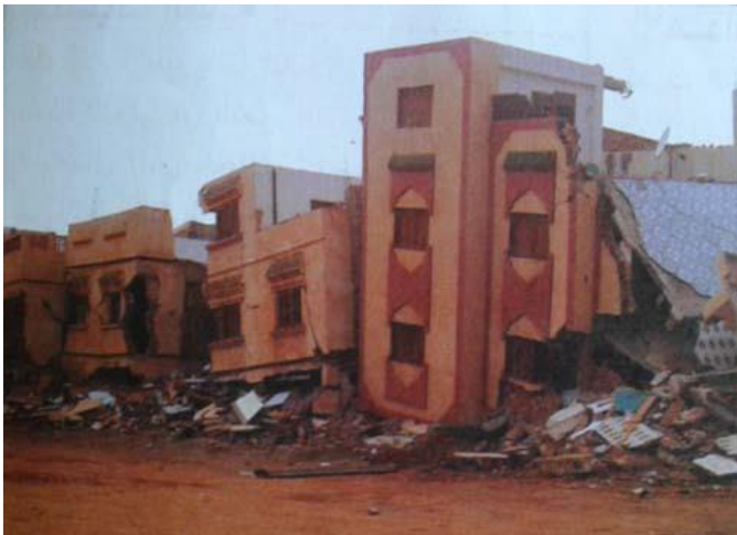
Picture 2. Earthquake Damage in Al Hoceima, 2004(p 16).
